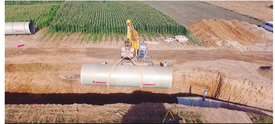
1 Main conveyance and network lines for irrigation Aydın Koçarlı-Irrigation of Bağarası DN3000-DN3400
