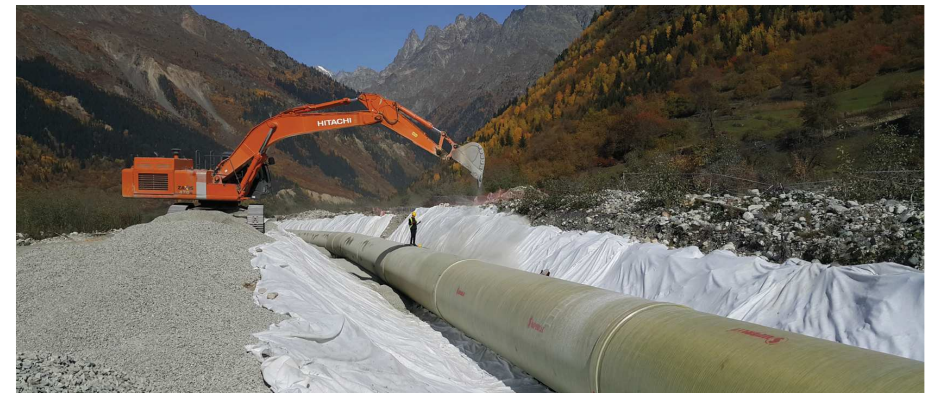
2 Mestia HPP Hydroelectric Power Plant DN 2400 / PN 6-10-16
